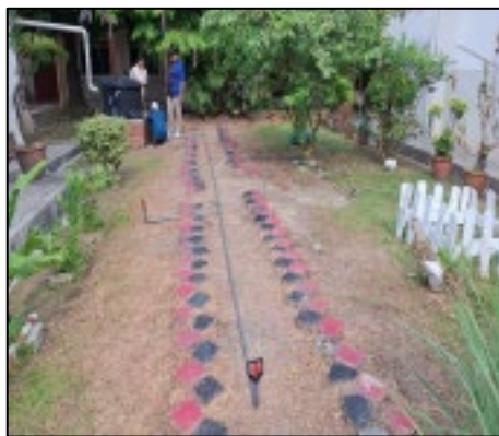
Rajah 1: Sprinkler irrigation system installed at the JPH
