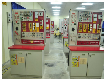
Electrical Machine Laboratory
