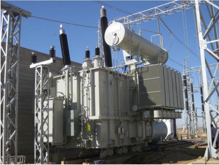
Figure 8 :High Voltage Transformer ( https://www.electricityforum.com/ )
