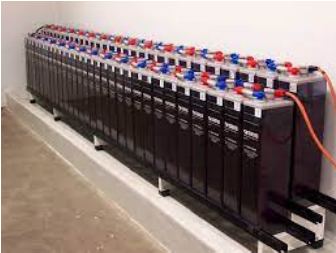
Figure 20 :Battery Bank ( https://www.tendersontime.com/ )
